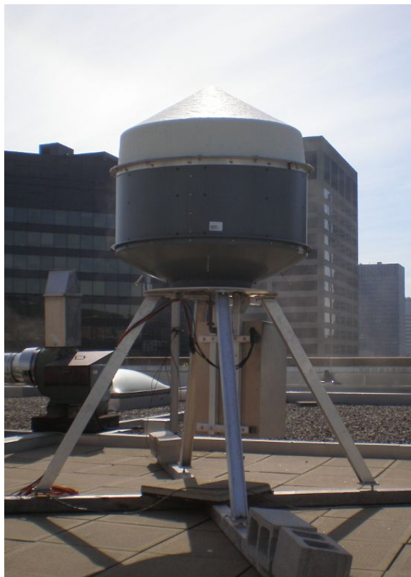
Figure 2: The Vertix Radar (Image source: McGill Vertix instrument webpage )
